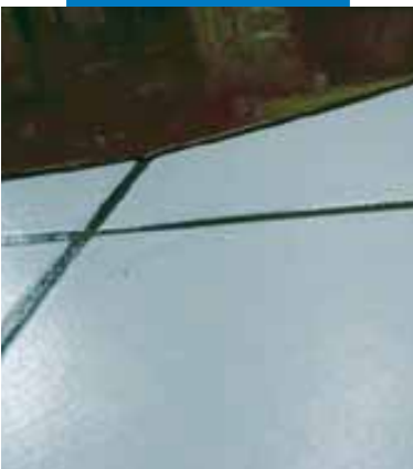
Detail of the application of Ultraplan on an existing ceramic tile floor after the application of Mapeprim SP
