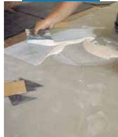
An example of an installation of inlaid PVC on a surface levelled with Ultraplan - CD2 - Milan - Italy
